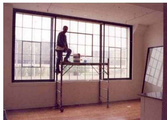
Storm windows can improve the efficiency of historic windows. These storm panels slide to allow the operation of the industrial windows.
