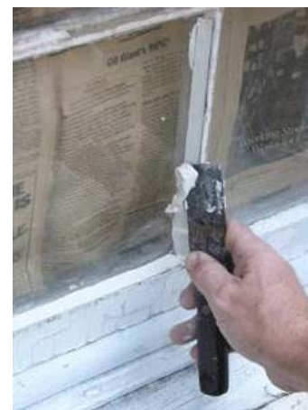
Some window repairs, such as reglazing, are relatively simple and perfect for do-it-yourself. More extensive repairs may require a professional.
