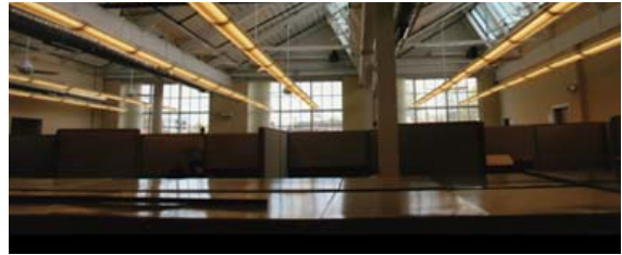
Historic buildings include many features, such as operating clerestory or cupola windows, designed to maximize ventilation and natural light.
